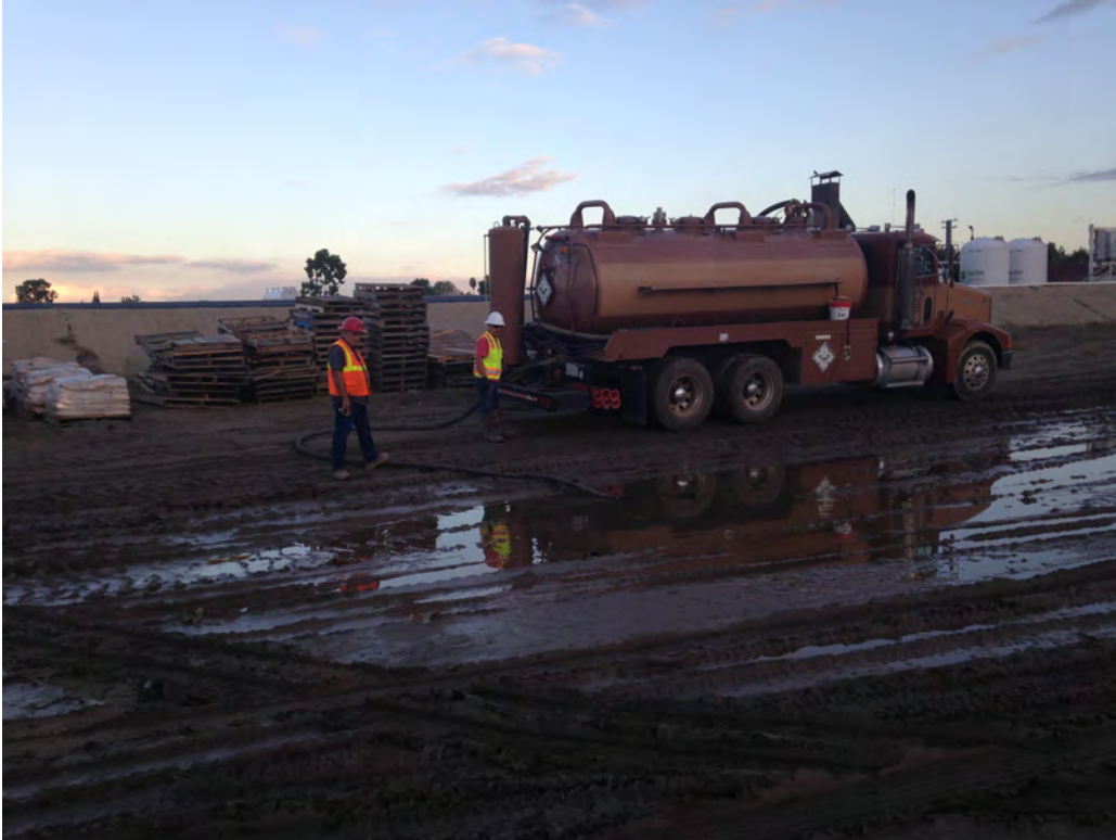
Photo 5: Vacuum truck used to extract ponding water post significant rain event, September 16, 2015.
